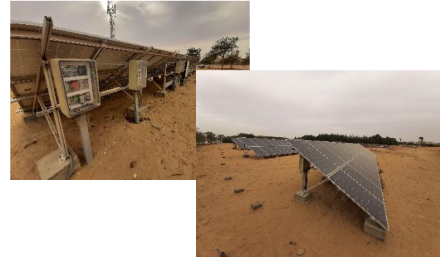
Maintenance and Operations Solar Plant
